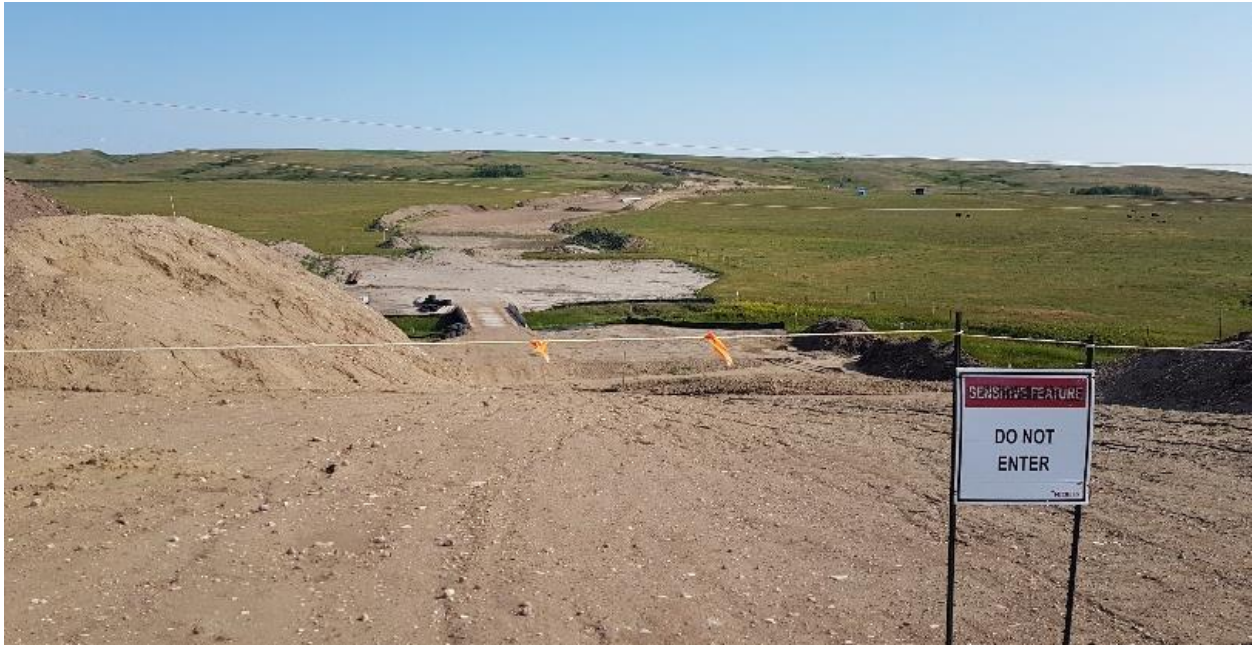
Figure 5 - Excavation site crossing a waterway in the Oyen area of southeastern Alberta
